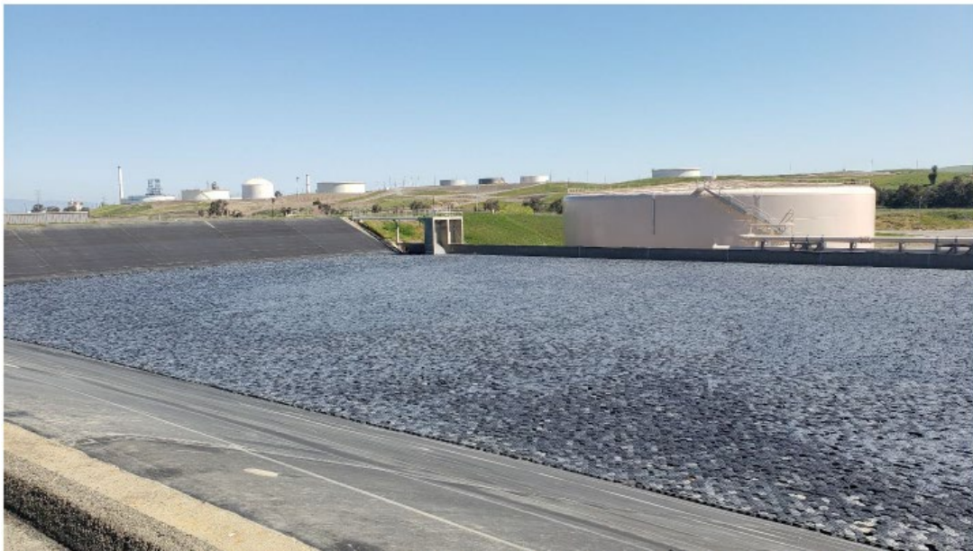
Photo 2: Another view of the west cell and the second new tank in the decommissioned east cell (north half of the reservoir).
